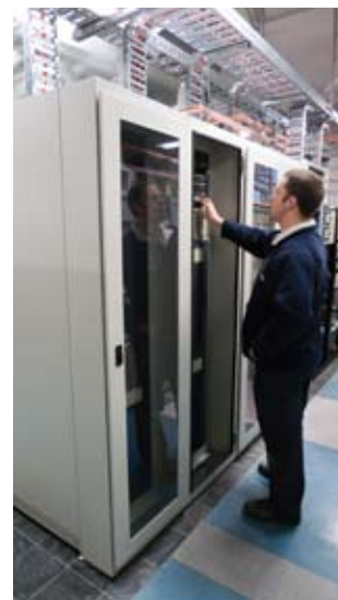
Adjusting the transmitter power in Melbourne: believed to be one of the highest-power DAB transmitter systems in the world to-date
